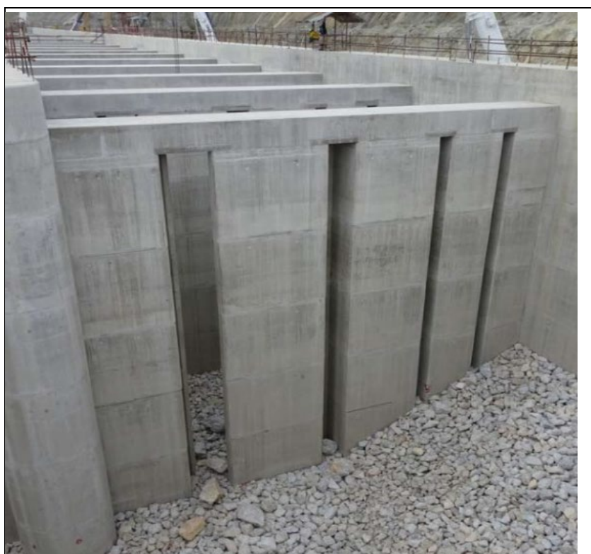
Figure 2: Vertical slot component of upstream fish pass (Source: Coe 2015 Xayabury HPP: Fish Migration Facilities, Pöyry and Fishtek [V1])
