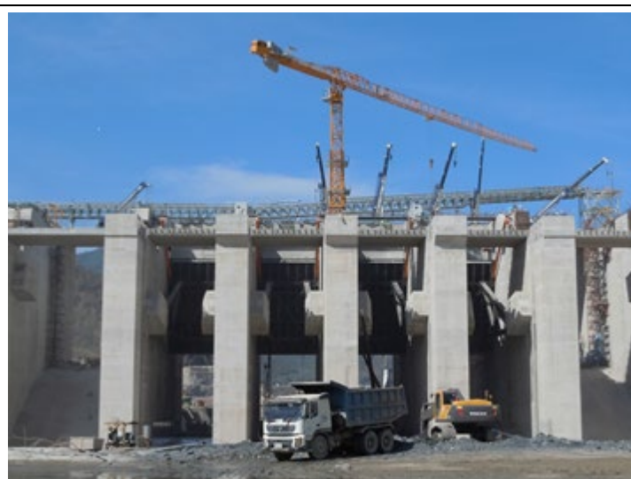
Figure A4.3: Low Level Spillway Gates under construction. Source: Poyry presentation July 2015
