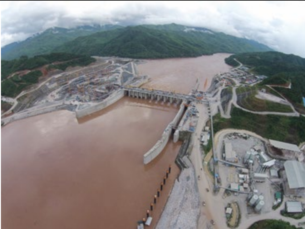
Figure 1: Aerial photo of Xayaburi construction site showing navigation lock (Source: Poyry presentation, July 2015)
