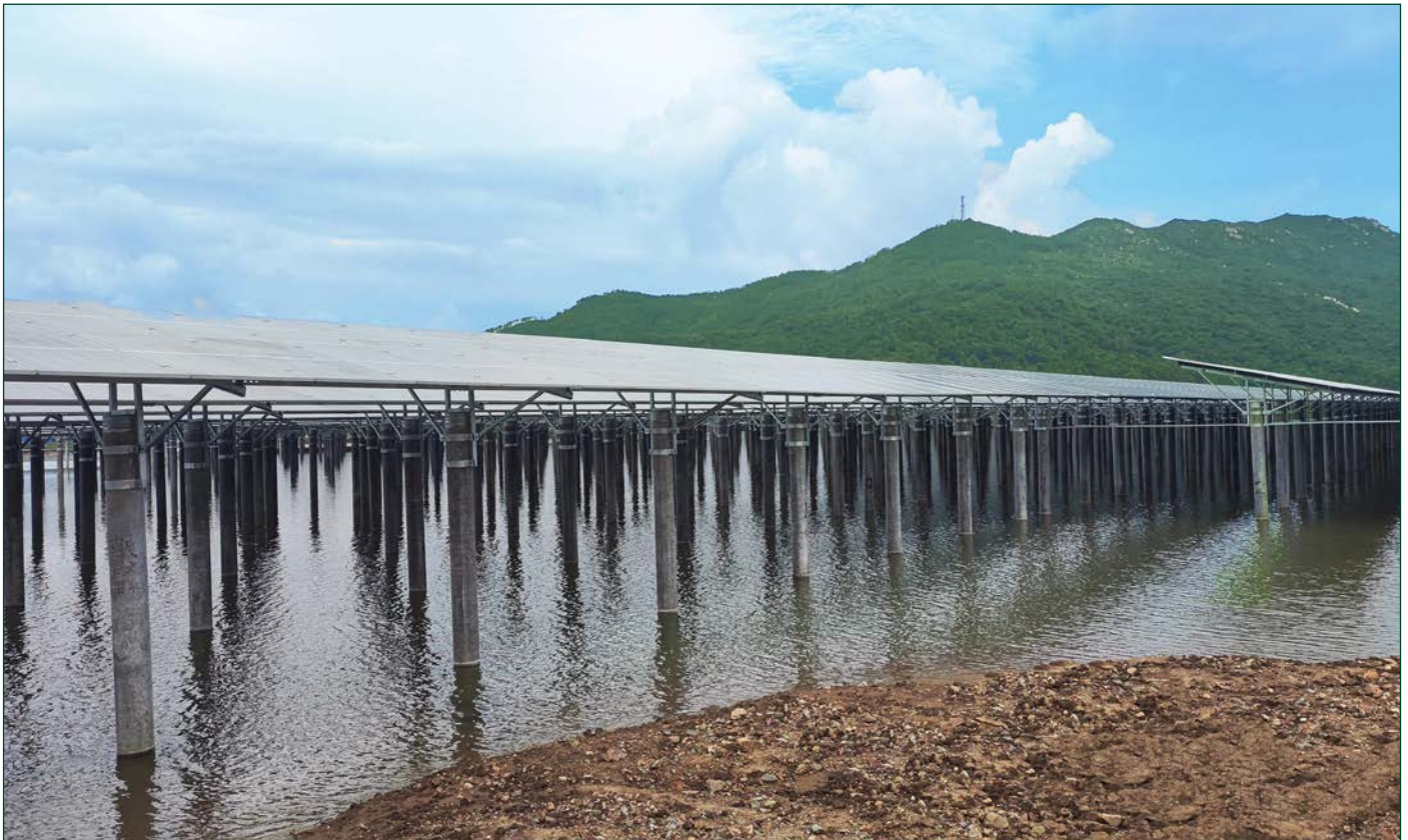
Photovoltaic system for ponds in Taishan in the Pearl River Delta
