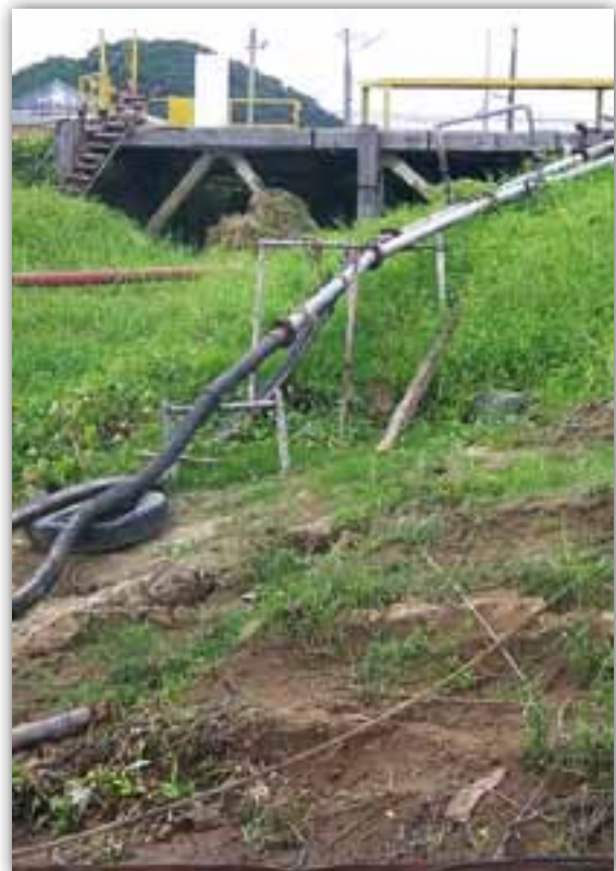
Figure 55: Cargo Pipes and Hoses Not Properly Supported
