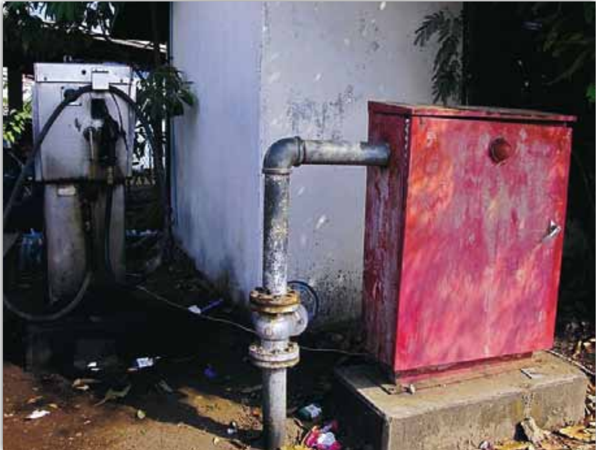
Figure 67: Poor Maintenance of Port Equipment
