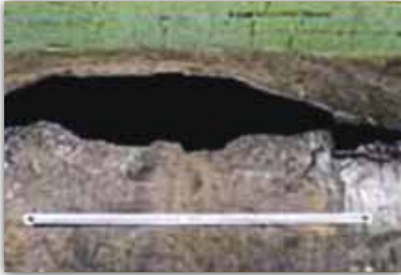
Figure 17: Corrosion Failure of Pipeline
