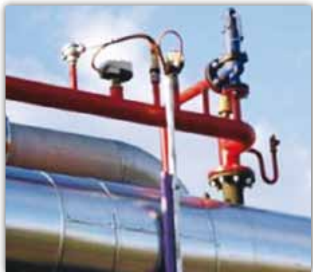
Figure 14: Pressure Relief Valve (painted blue)
