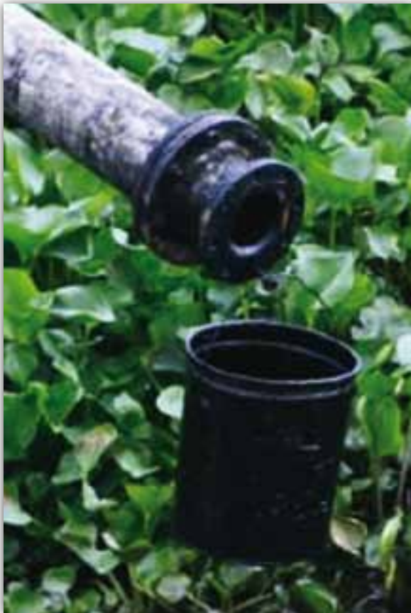
Figure 15: Cargo Line Not Blinded
