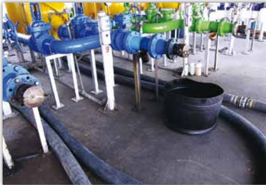
Figure 60: Cargo Pipes Not In Use Not Fully Bolted
