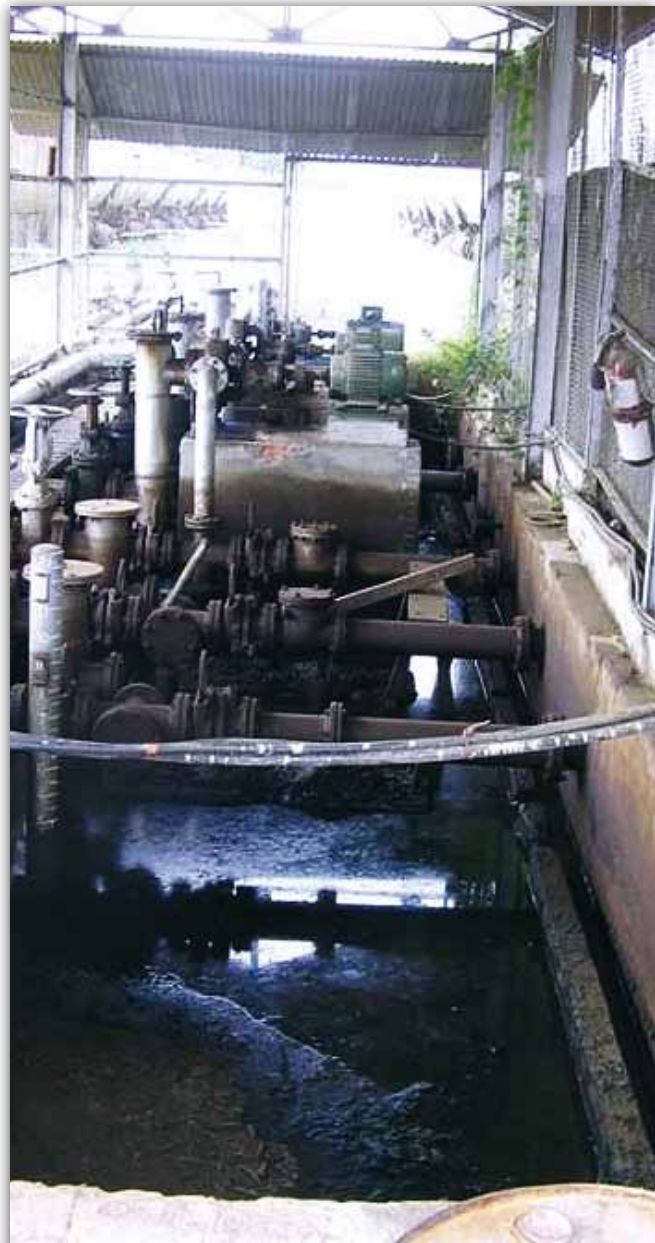
Figure 53: Poorly Maintained Equipment
