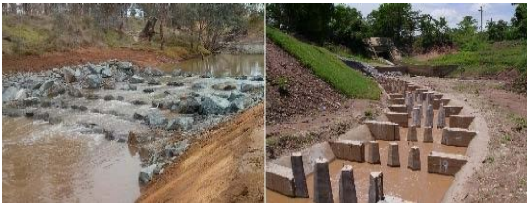
Figure 25: A full-width rock-ramp fishway (left) will provide fish passage over all flows, while a partial width fishway (right) can only operate on a low range of flows.
