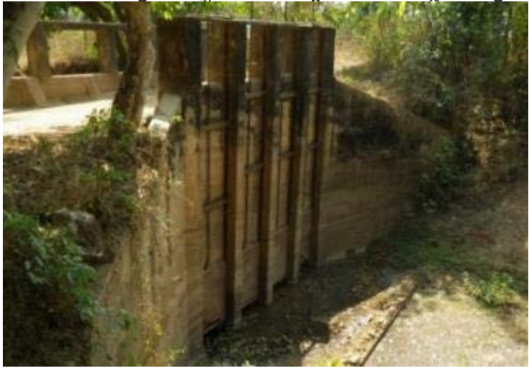
Figure 33. Steel regulator gates controlling water on a wetland outlet.
