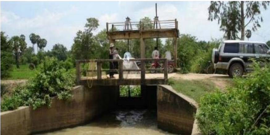
Figure 34. Another steel regulator gate controlling water from a wetland under a road crossing.
