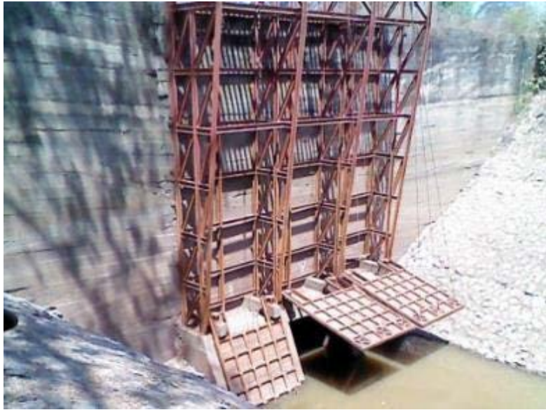
Figure 35. Floodgates on the outlet to wetlands in the Xe Bang Fei system.
